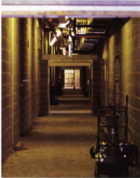
Service corridors at Paddington Central, underneath the roof deck
