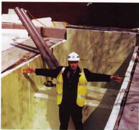
The author demonstrates where the tree sand should go, prior to soiling at Paddington Central
